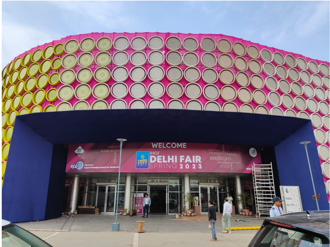
PHOTO - 3 - Overview of 55th IHGF Delhi Fair Spring'23 - Construction is in full swing at India Expo Mart, Greater Noida.
